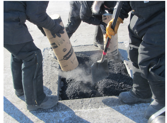
Above: Thanks to iHMA's induction heating method, asphalt repairs can now be made in any weather condition—including freezing or even sub-freezing temperatures.
